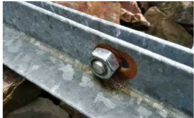
A galvanised washer and a stainless steel nut have caused a poor surface ratio (source: OBO Bettermann)
