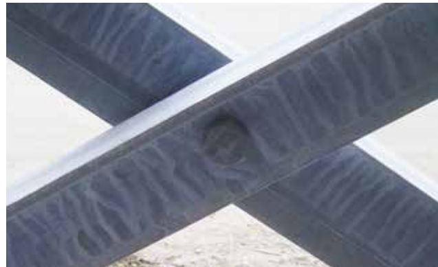
Light white rust on a hot-dip galvanised construction (source: Institut Feuerverzinken)
