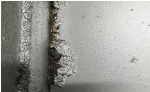
Gap corrosion on an enclosure. The increasing under-rusting damages the coating (source: OBO Bettermann)
